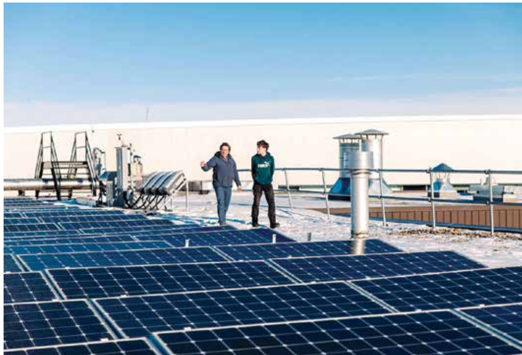
The campus features nearly 4,200 solar photovoltaic panels with an installed capacity of 1.6 MW, notably including the largest institutional solar array in Canada.
