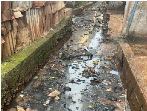
The sewerage system in Kroo Bay.
