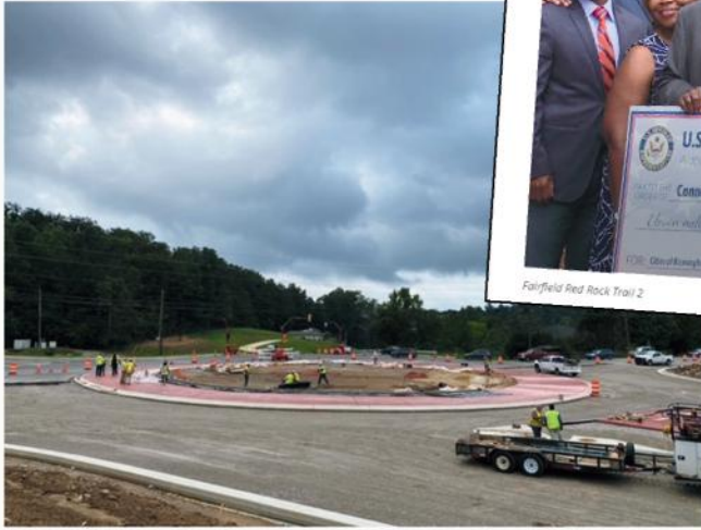
Photo of the new roundabout taken last Friday (Photo provided by Helen Hays)
