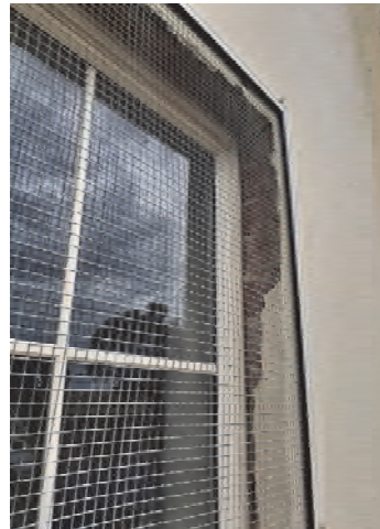
Render to be repaired
