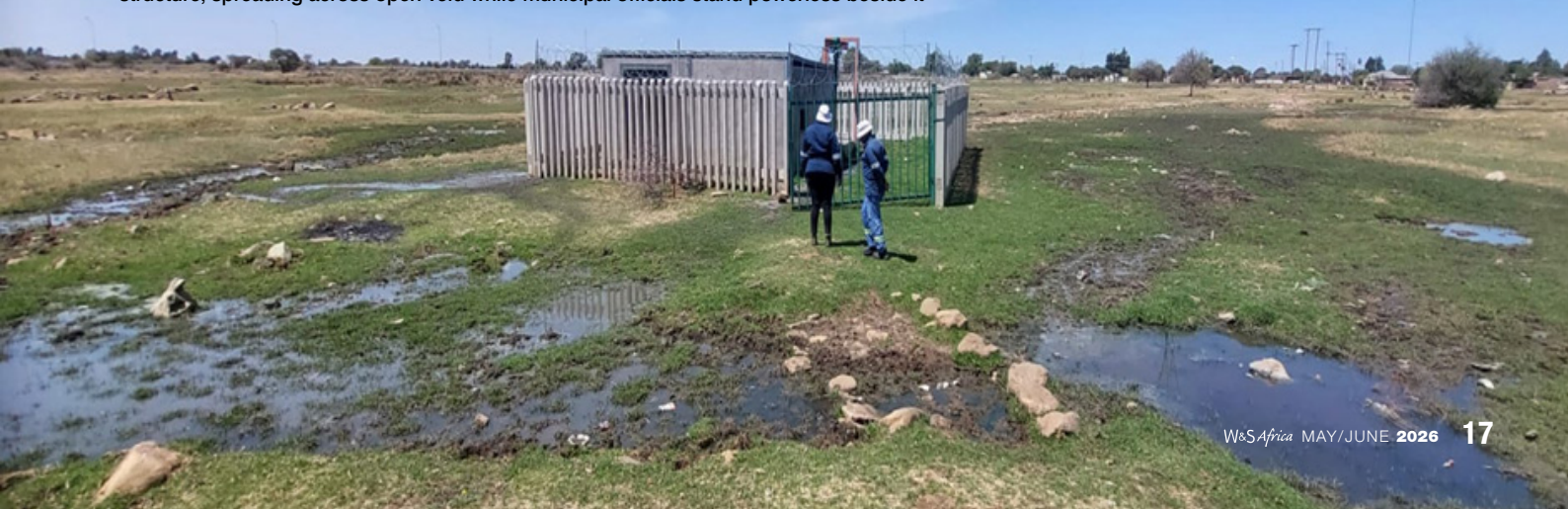
Warrenton N12 Pumpstation: Raw sewage overflows from a collapsed pump station structure, spreading across open veld while municipal officials stand powerless beside it
