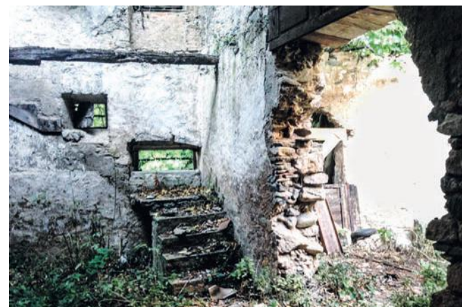
Some of the buildings were a total ruin when they bought their 'ugly duckling'
