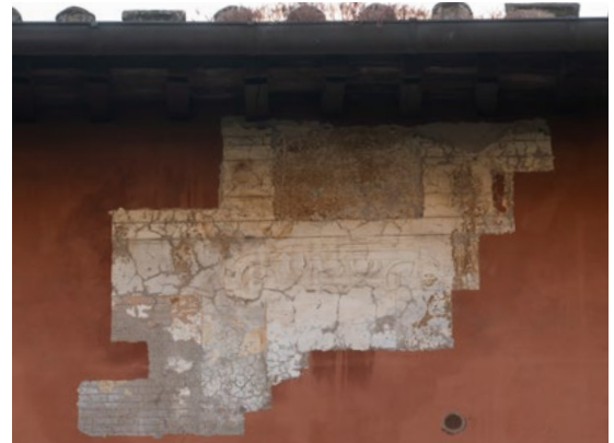
First painted Ionic column and surrounding brickwork uncovered by the renovation team
