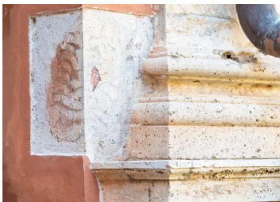
An example of the layers of history found in the cloister, carefully peeled back as part of the preparatory work for the cloister renovations.
