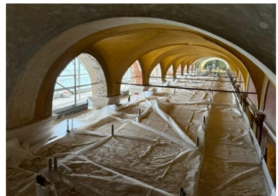
The arches of the cloister walkway, above the scaffolding, are being stripped down to the original plaster and then painted in their original colors.
