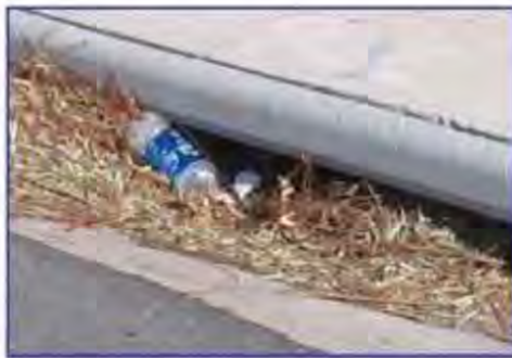
Blockage of vegetation and trash
