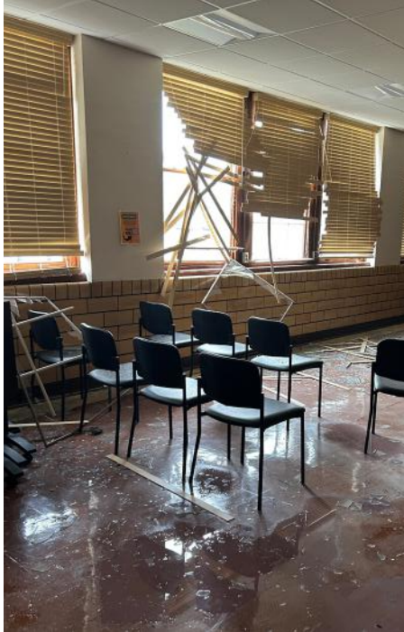
The board meeting room in the old high school was left uninhabitable after the tornado, with shattered windows, broken glass, and significant water damage throughout the space.
