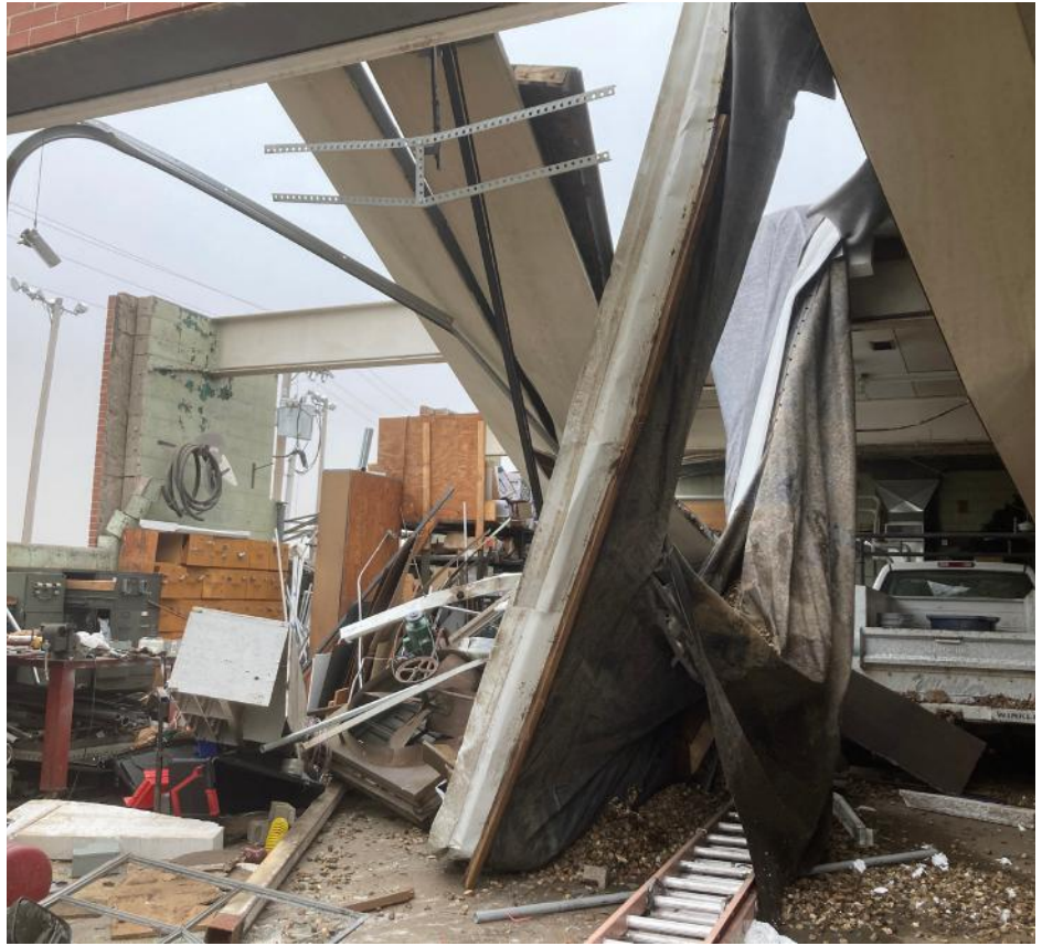
Sections of the maintenance and IT facility collapsed into work areas, crushing equipment and vehicles under twisted metal and debris.
