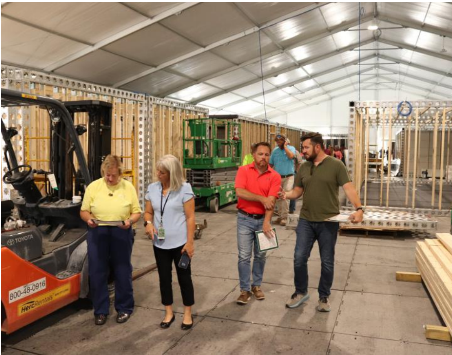
Superintendent Dr. Fara Jones (center, in blue) joined district leaders and board of education members on-site to review progress and ensure the temporary school would be ready for students.
