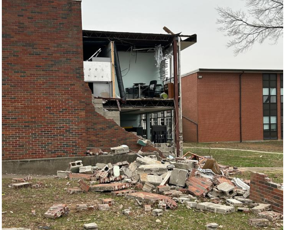
The high school experienced severe damage to the roof and wall, exposing classrooms and leaving piles of brick and debris scattered across the grounds.
