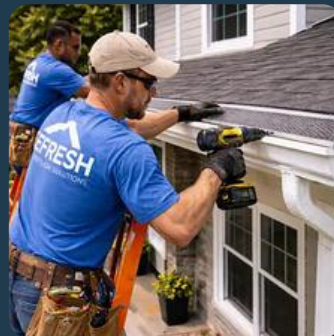
Gutter & Gutter Protection
