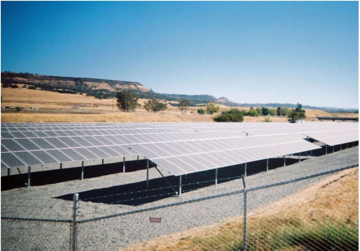
One of two solar arrays that power the Butte County Administration Building. Photo courtesy of the Butte County Department of Development Services.
